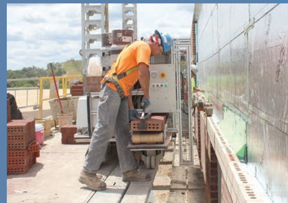
Semi-Automated Mason, or SAM, a brick-laying robot created by New York-based Construction Robotics
